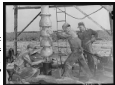
Getting ready to put in the pumping part of the water well for irrigation purposes on a farm near Garden City, Kansas. September 1939. LC-USF34- 034141-D
